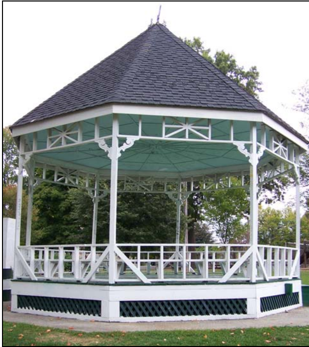
Existing gazebo – to be replaced because it's deteriorated and beyond simple repair.
