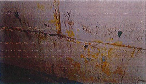
Mold growth on back-side exterior wall in the Weight Room
