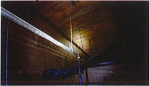
View above ceiling tiles in the Fire Dept (Sleeping Quarters / Restroom); surfaces have been sealed with foam
