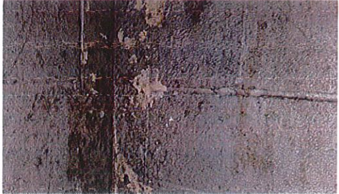
Mold growth and signs of water infiltration through walls in the Hose Tower
