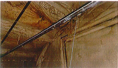
View above ceiling tiles in the Fire Dept (Sleeping Quarters / Restroom); surfaces have been sealed with foam
