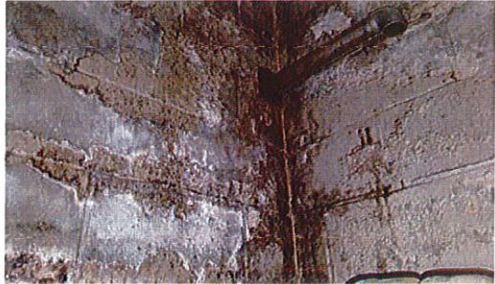
Mold growth and signs of water infiltration through walls in the Hose Tower
