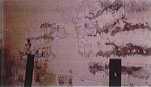
Signs of water infiltration through the back-side exterior wall in the Weight Room
