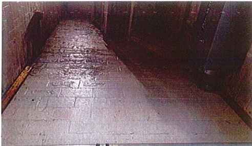
Water infiltration appears to be occurring high up in the Hose Tower, possibly at the interface with the roof of the truck Bay
