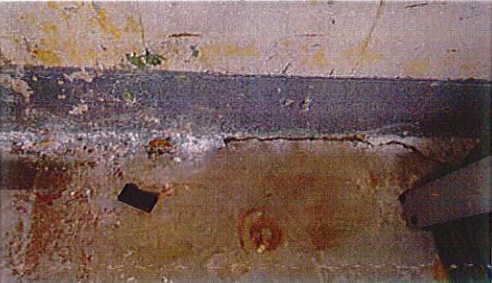
Signs of water infiltration through the back-side exterior wall in the Weight Room
