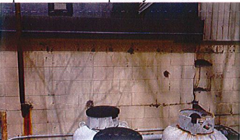
Damage to wall system at back-side of building (outside of the Fire Dept)
