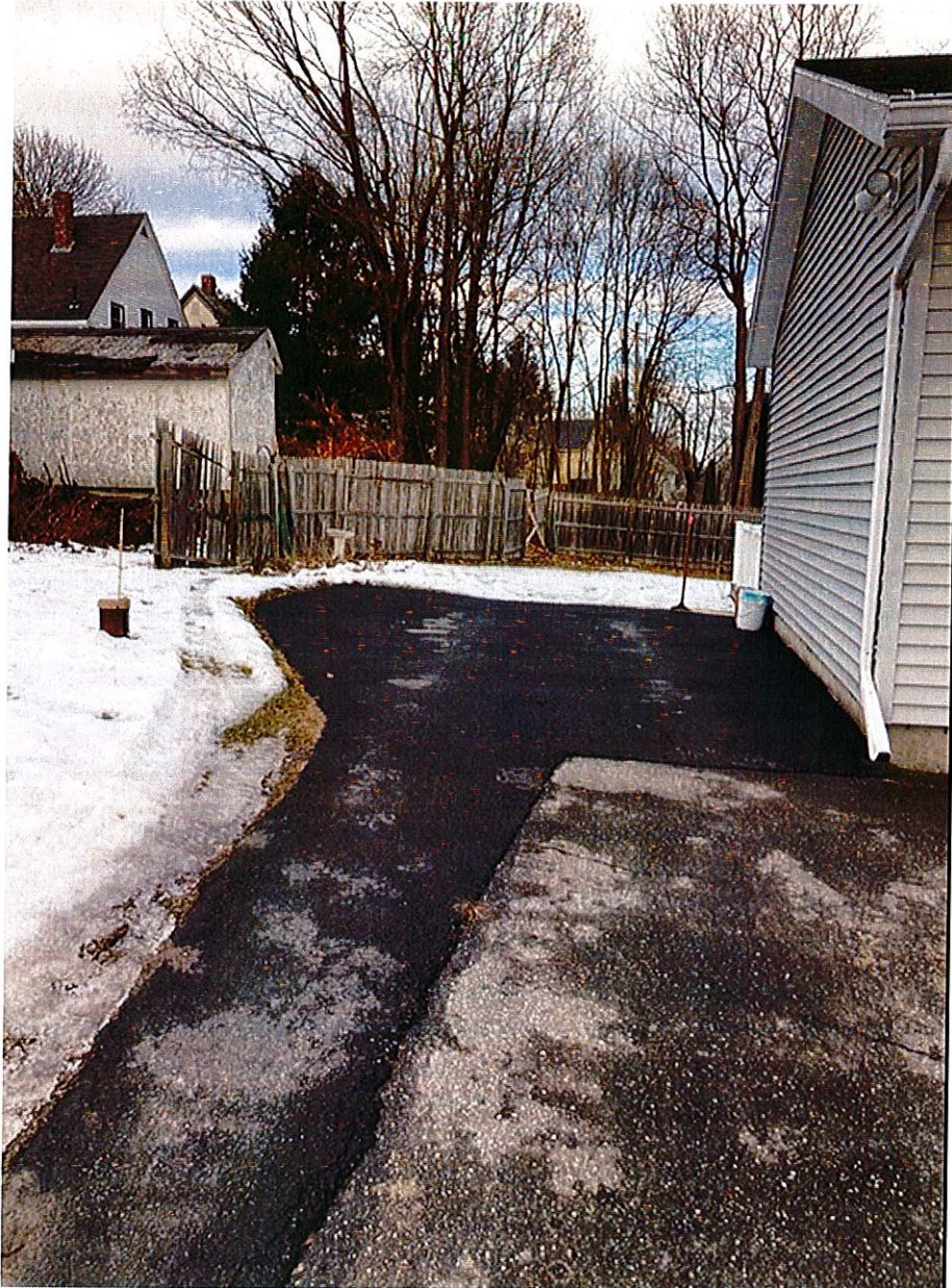
View of proposed garage area with pink marker showing 32" space for walk through.
