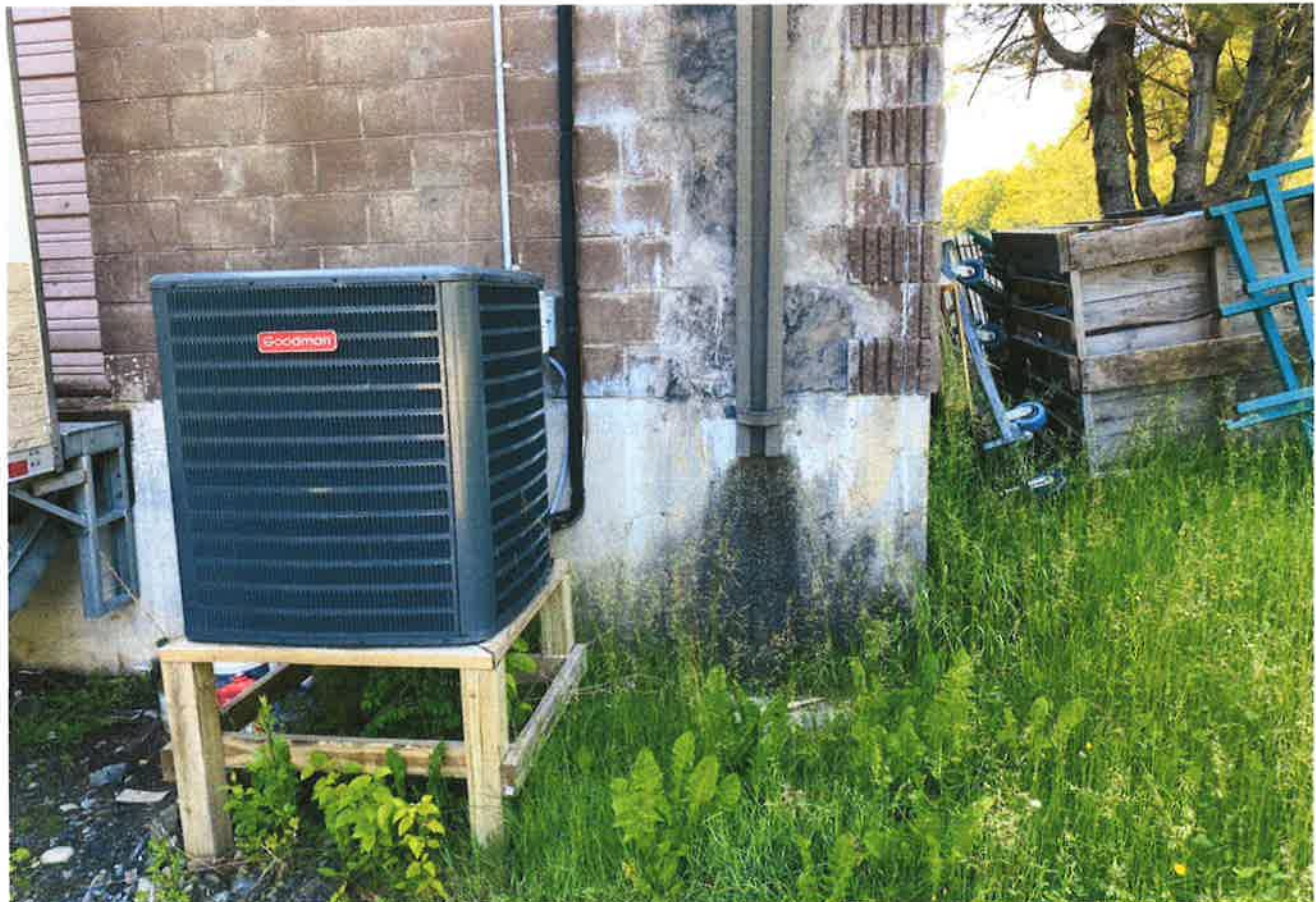
another air conditioning unit on street end of bulidng
