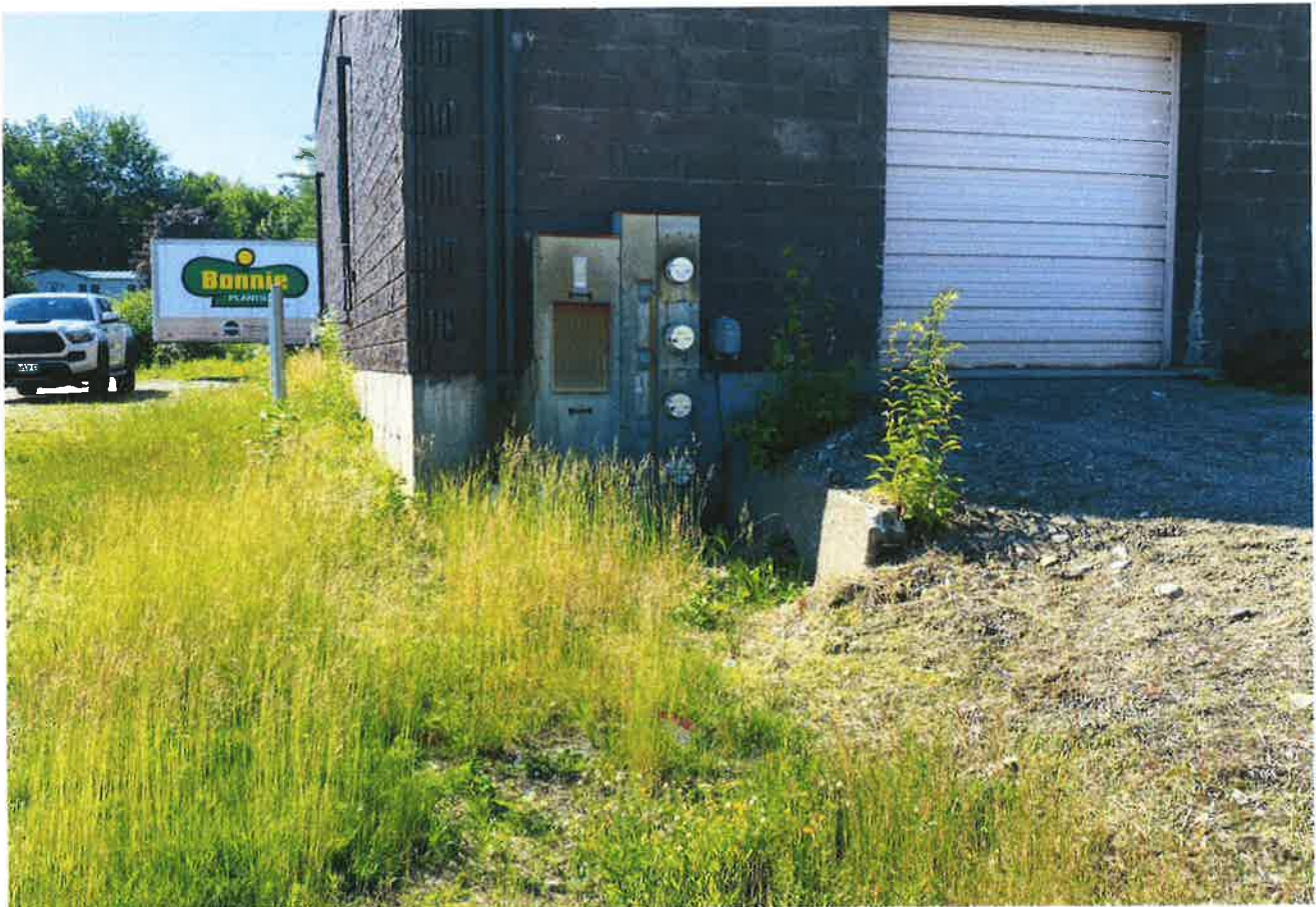
Electrical entrance at corner of building
