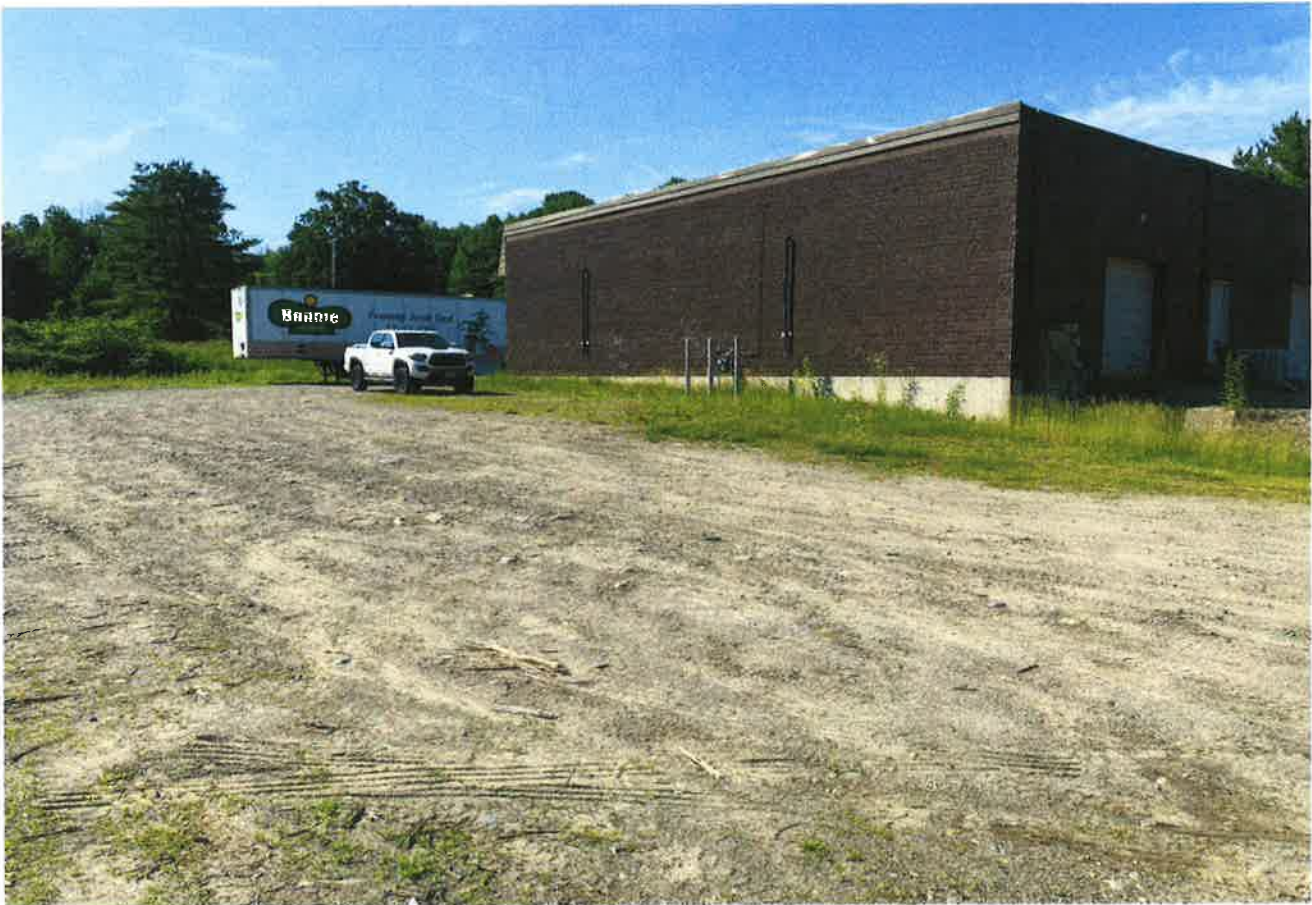
side yard building elevation gas meeter with bollards
