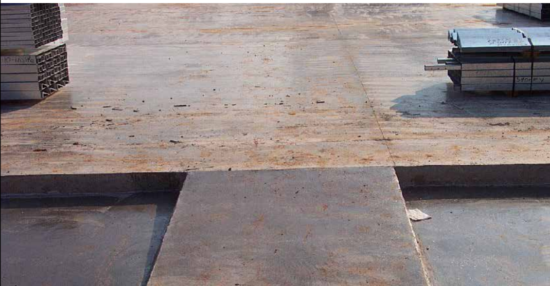
This ramp started at the top of the step and slopes at a 1":12" slope to the lower finished floor.
