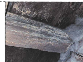
PHOTO 9 MOLD ON FRAMING MEMBERS
