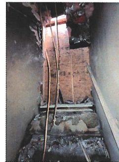
PHOTO 4 SEPARATION OF THE MASONRY WALL FROM THE BUILDING
