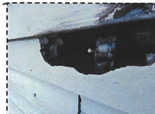
PHOTO 6 CLOSEUP VIEW OF REAR EXTERIOR BEARING WALL NOTE CONDITION OF WALL FRAMING AND LACK OF WALL SHEATHING DUE TO FIRE
