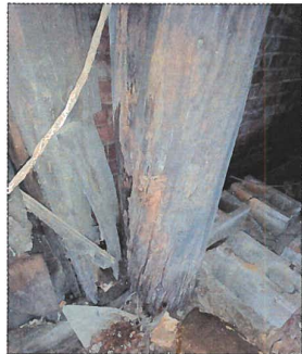
PHOTO 8 DRY ROT LOG SUPPORT POST
