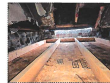
PHOTO 5 SEPARATION OF THE MASONRY WALL FROM THE BUILDING
