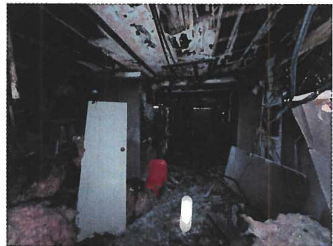
PHOTO 6 APARTMENT 8 SUSTAINED MASSIVE FIRE DAMAGE
