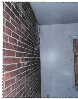
PHOTO 4 INTERIOR VIEW OF IN APARTMENT 11 NOTE EXISTING EXTERIOR MASONRY WALL IS INTACT
