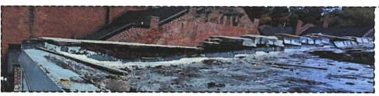
PHOTO 5 VIEW OF NORTHEAST CORNER OF ROOF NOTE CONDITION OF REMAINING PARAPET, FLASHING, AND ROOF MEMBRANE. NOTE FIRE DEBRIS BLOCKING ONLY ROOF DRAIN.
