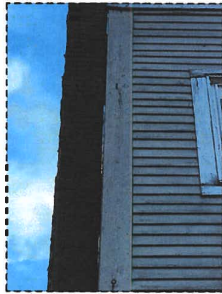
PHOTO 7 VIEW OF NORTHEAST CORNER OF BUILDING UNIT NOTE MASONRY WALL IS SEPARATING FROM WOOD FRAMED STRUCTURE.
