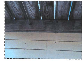
PHOTO 8 VIEW OF FIRE ESCAPE LEDGER ATTACHMENT NOTE CONDITION OF REAR WALL NEGATES THE STRUCTURAL CAPACITY OF THIS ATTACHMENT
