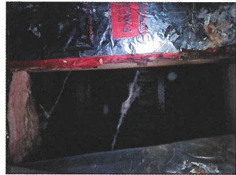
PHOTO 2 ROOF MEMBERS COMPROMISED BY FIRE NOTE THE EXTENSIVE SMOKE DAMAGE
